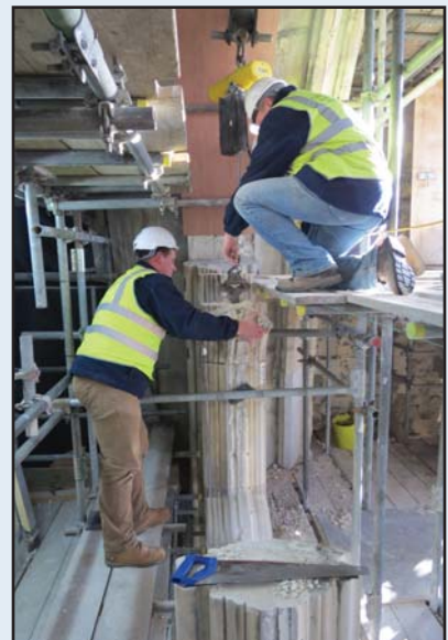
Dismantling the tracery at the top of the Great South Window - very carefully.
